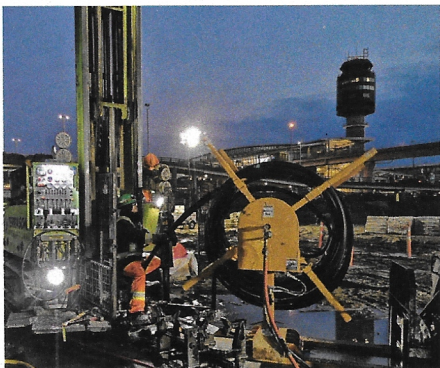
3. Each of the boreholes at Vancouver International Airport contains 1,000 feet of 1.25-inch PE4710 high-density polyethylene (HDPE) pipe. Courtesy: PPI
