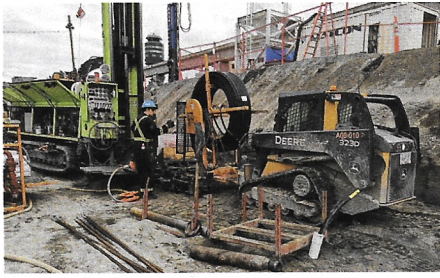
2. The piping loop, after being placed in the ground, was surrounded with thermally enhanced grout. Courtesy: PPI
