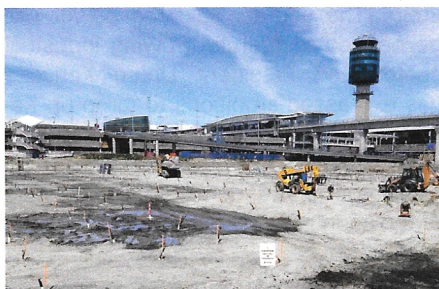
1. The Vancouver airport's system required hundreds of vertical boreholes to provide sustainable heating and cooling for the terminal. It is one of the largest geothermal energy projects in Canada. Courtesy: Plastics Pipe Institute (PPI)
